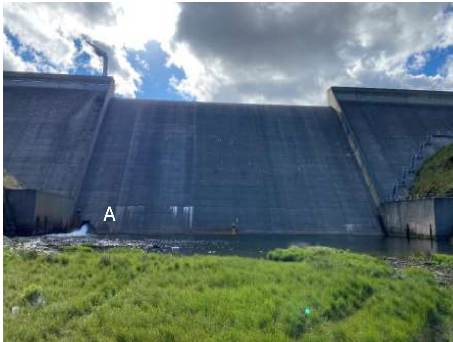
Figure 1-1 Tantangara Dam wall pictured from downstream. The outlet valve can be seen at the lower left of the wall (A).
